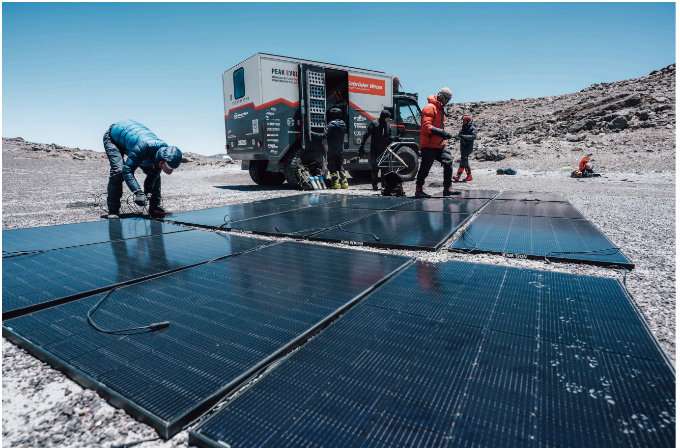
The team setting up the solar power plant at base camp. Altitude: 6,200 metres above mean sea level (Photo credit: Anna Plocinska)
